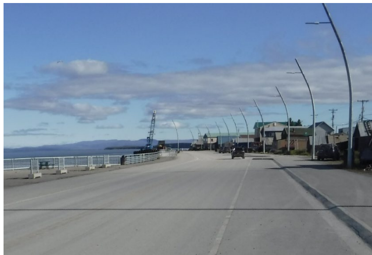
Improvements to Shore Avenue including pavement, cultural placards, and a scenic viewing area, Bristol 2017
