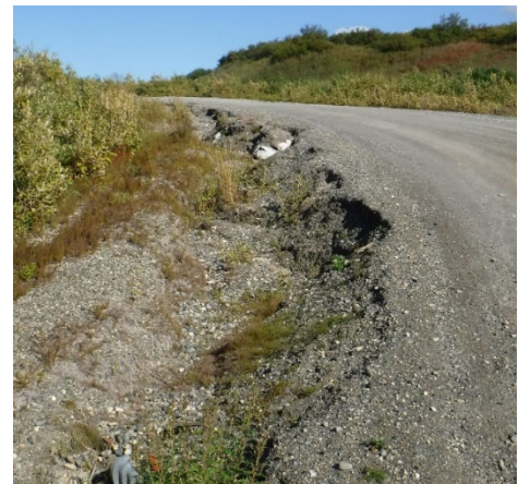
Shoulder erosion on Air Force Road, Bristol 2017
